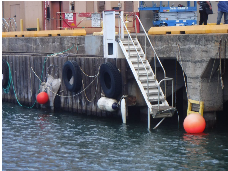
Photo 4: Stairs to be Replaced
